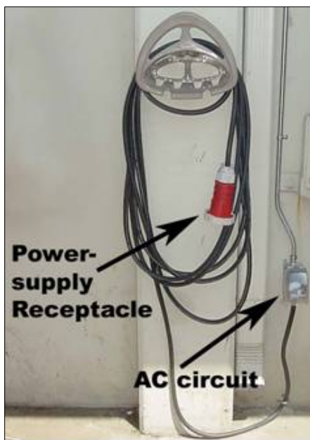
Figure 5: Receptacle and power supply.
