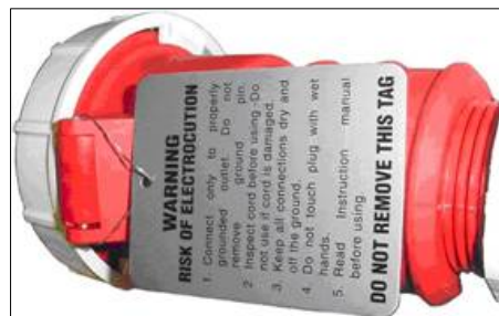
Figure 11: Power-supply receptacle with warning tag.
