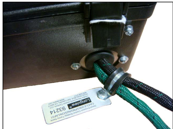
Figure 4: CARB-verification label attached to wiring harness at Controls Box. (Example is from a Longview system.)
